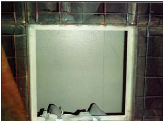
Clean Back Plenum
